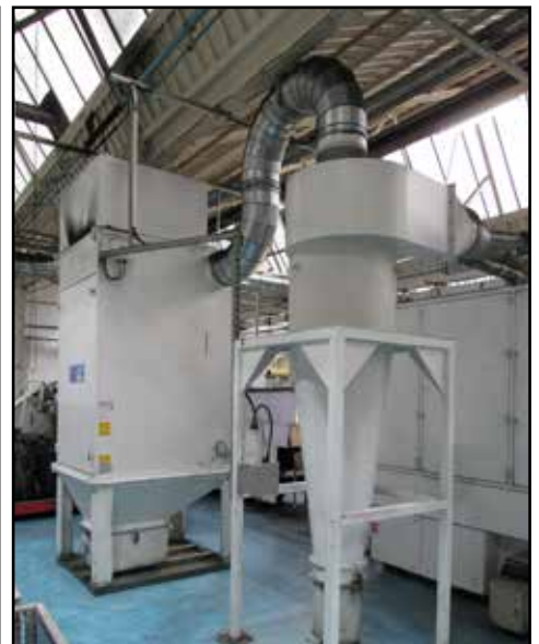
DUST CONTROL SYSTEMS CYCLONE & SHAKEDOWN
