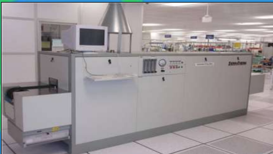
SIERRATHERM CLEAN ROOM TUNNEL OVEN
