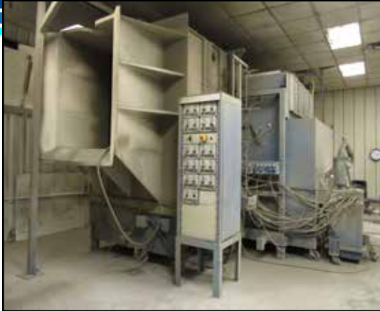
NORDSON POWDER PAINT BOOTH
