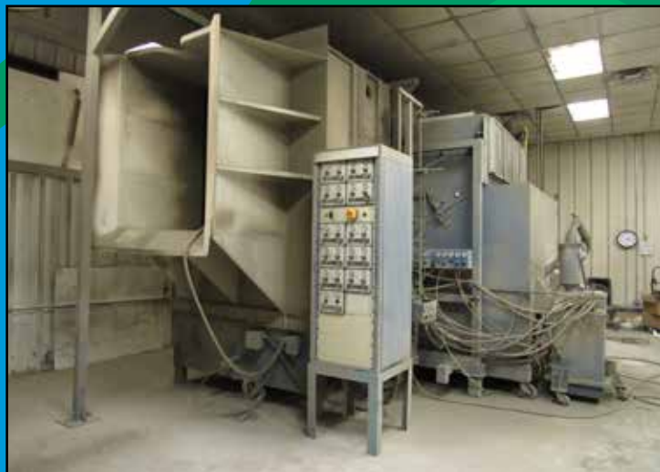
NORDSON POWDER PAINT SYSTEM
