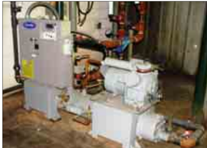
CARRIER 40 HP AIR COMPRESSOR
