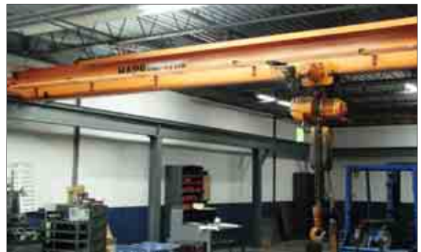
HARRINGTON 5 TON BRIDGE CRANE WITH PENDANT CONTROL
