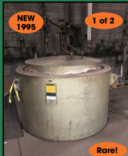
LINDBURG "PIT-TYPE" HOMO TEMPERING FURNACE
