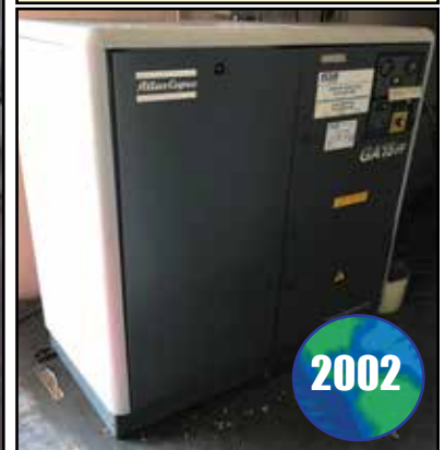
ATLAS COPCO ROTARY SCREW COMPRESSOR
